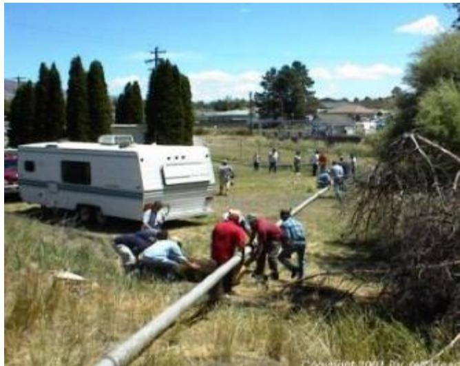
Farmers and their supporters lay pipe to pump water around head gates
